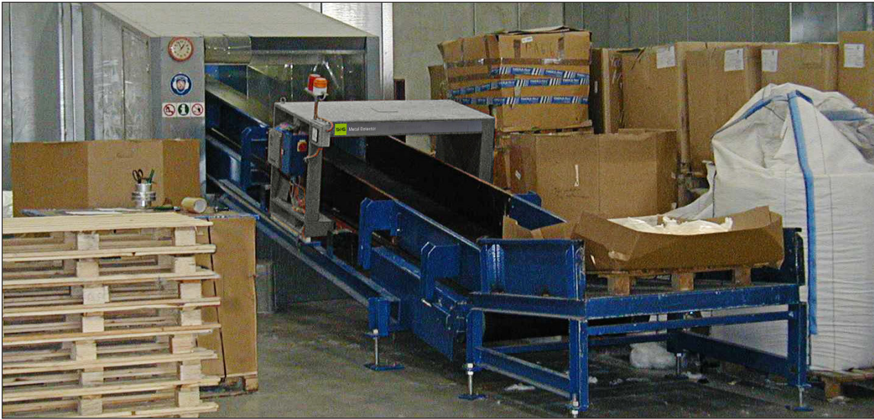
Installation example: Tunnel metal detector DLS analysing recycling material before the granulator. (old version)
